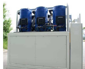
Enefcogen 30kW System
